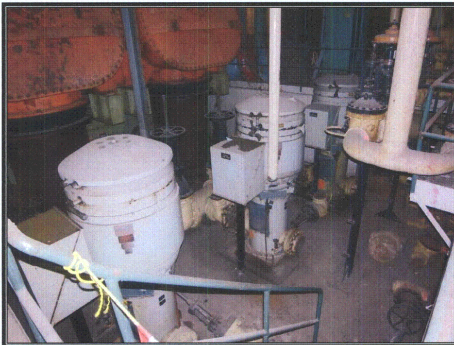
Plate 24 Condensate pumps (Photograph by RCG&A, 2008)
