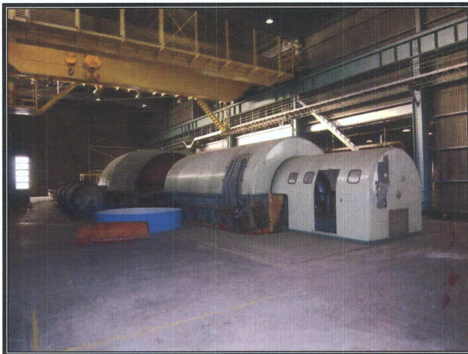
Plate 27 Turbine generator looking northwest (Photograph by RCG&A, 2008)
