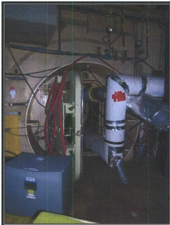
Plate 63 Inner personnel access door (Photograph by RCG&A, 2008)
