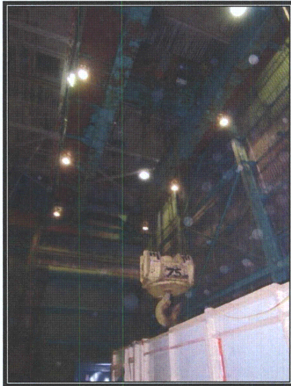
Plate 121 Overhead crane in FARB (Photograph by RCG&A, 2008)
