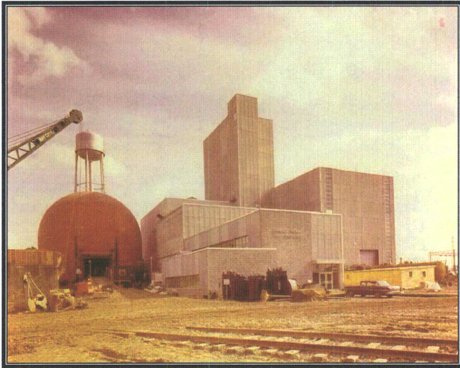
Plate 69 View looking east showing temporary opening in reactor containment building (Courtesy DECo)
