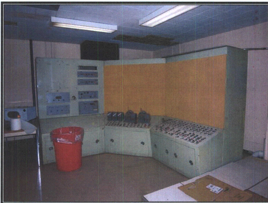
Plate 37 Remote control panel for reactor building crane (Photograph by RCG&A, 2008)
