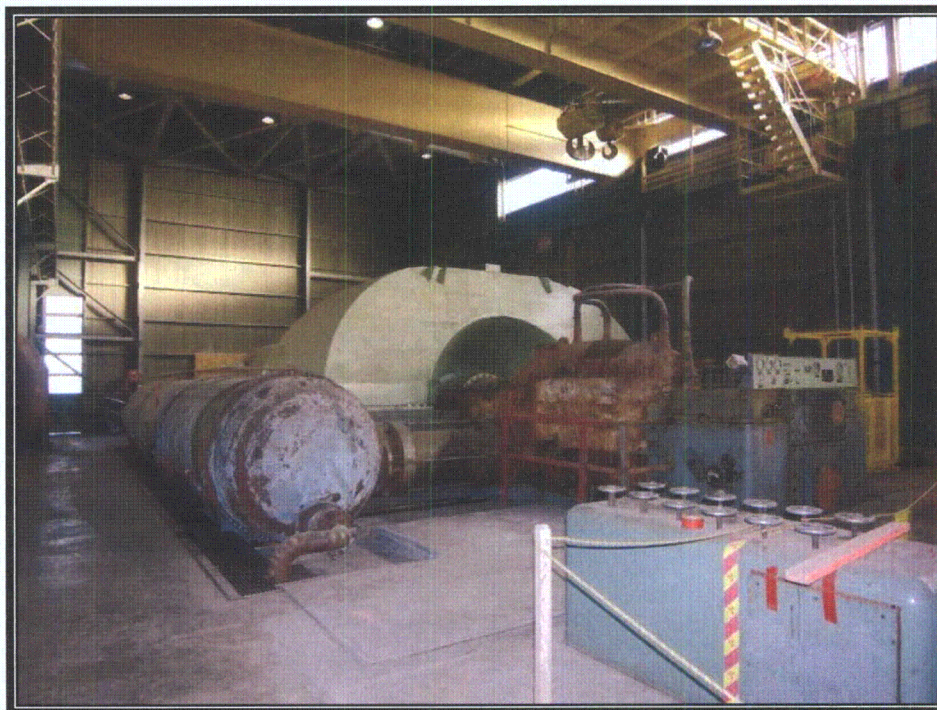
Plate 28 View of turbine generator showing re-heaters (Photograph by RCG&A, 2008)
