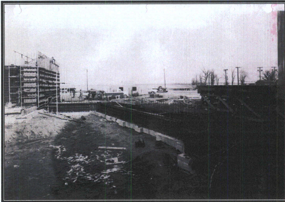
Plate 78 Construction photograph of primary sodium gallery, note sodium service building in background (Courtesy DECo)
