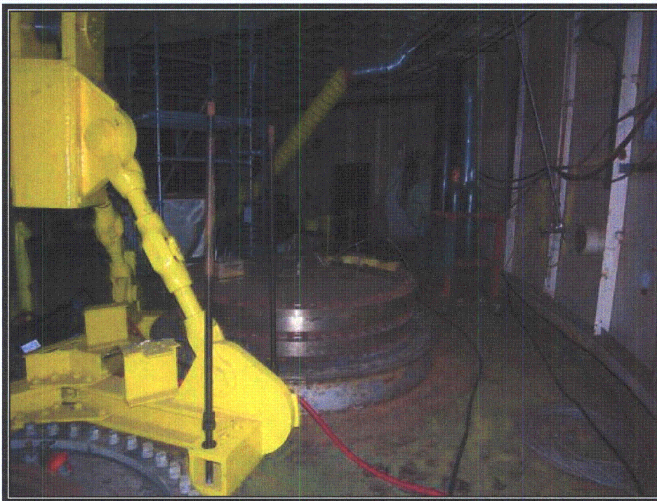
Plate 83 Location of intermediate heat exchanger (Photograph by RCG&A, 2008)
