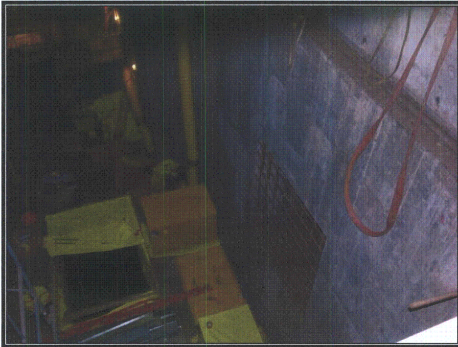
Plate 115 Opening for ledged glass window (not installed) in repair pit (Photograph by RCG&A, 2008)
