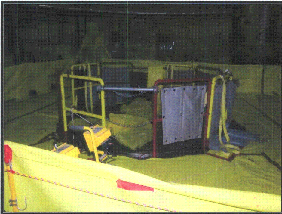
Plate 81 Top of reactor vessel (Photograph by RCG&A, 2008)
