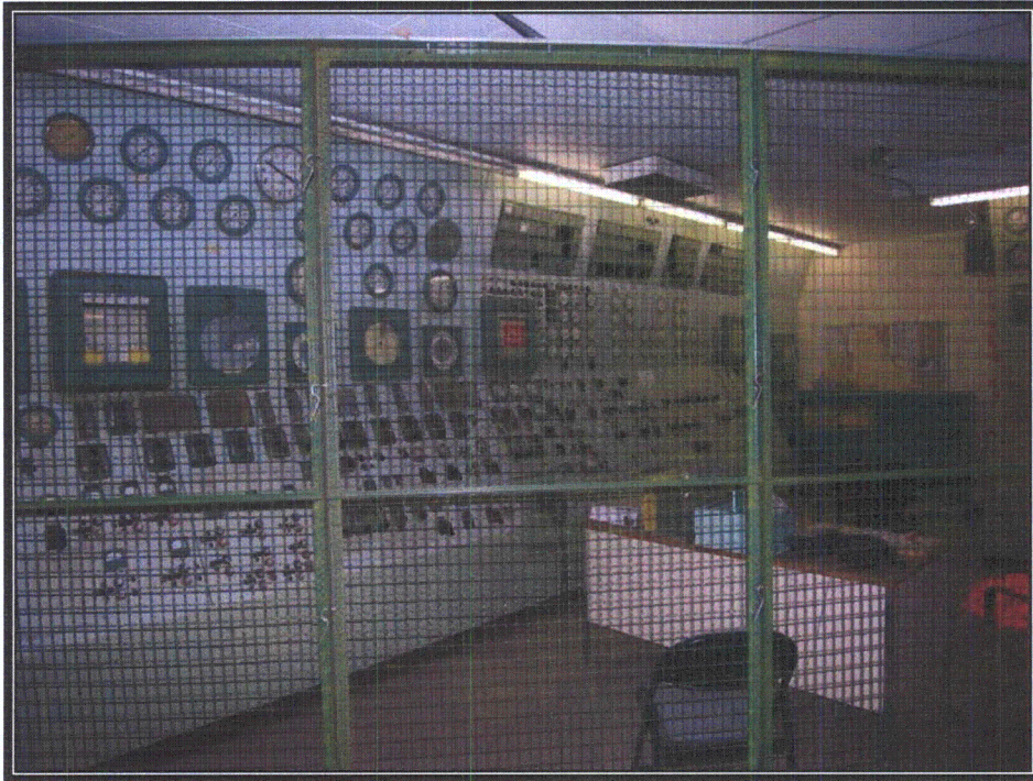
Plate 42 Auxiliary panel for peaking boiler (Photograph by RCG&A, 2008)
