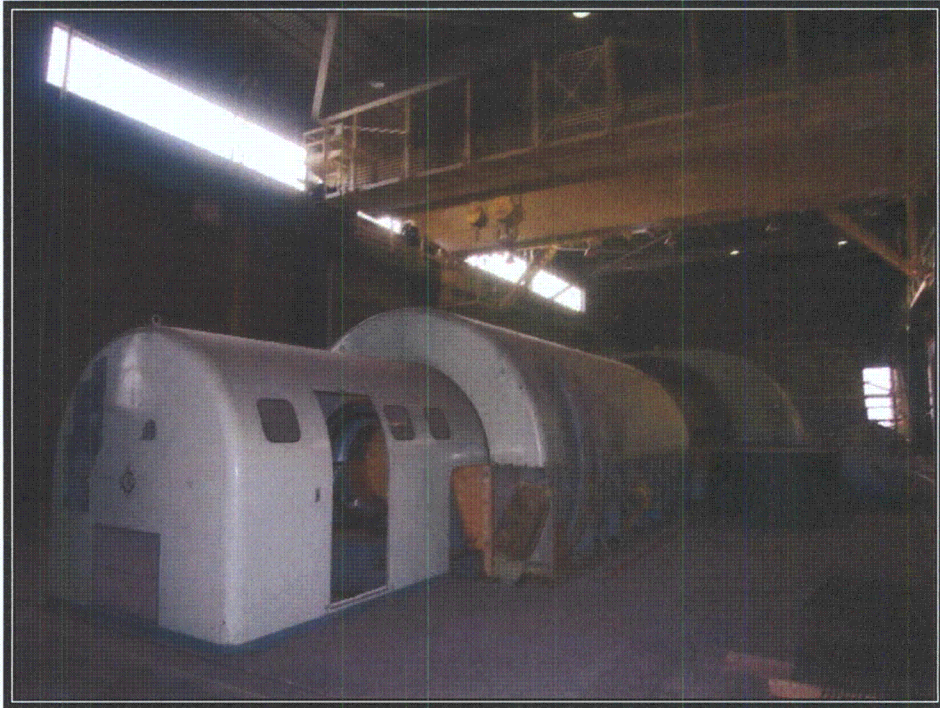
Plate 29 View of turbine generator looking southwest (Photograph by RCG&A, 2008)
