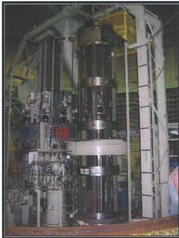
Plate 174 Top of reactor. The offset handling mechanism is in front and the hold down device and control/safety rods to the rear (Courtesy DECo)
