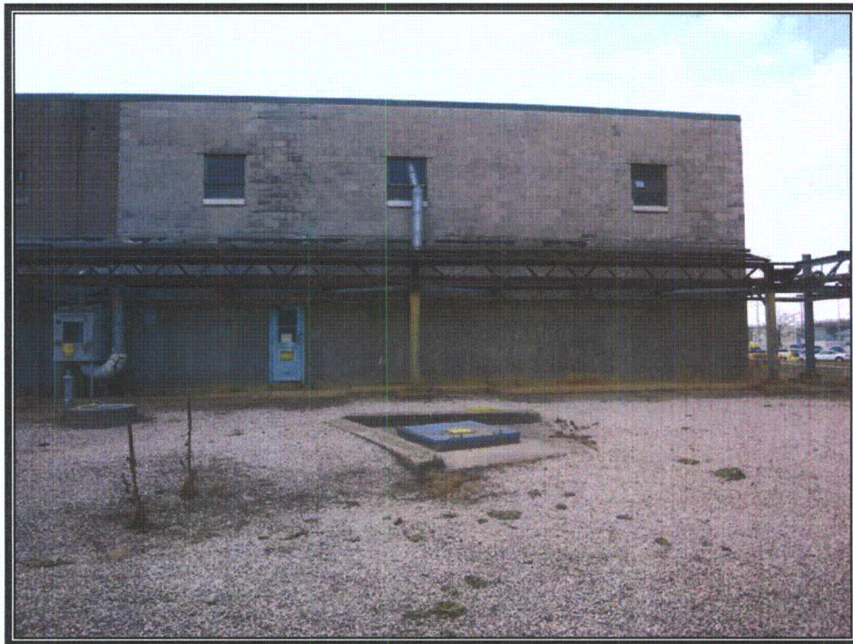
Plate 136 East wall of sodium service building showing upper, concrete block section (Photograph by RCG&A, 2008)
