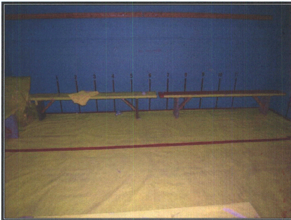
Plate 132 Index marks on wall of new fuel storage room (Photograph by RCG&A, 2008)
