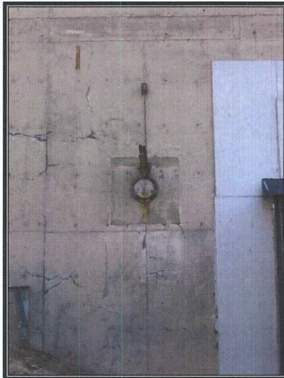
Plate 141 Reinforced instrument port in north wall of sodium service building (Photograph by RCG&A, 2008)
