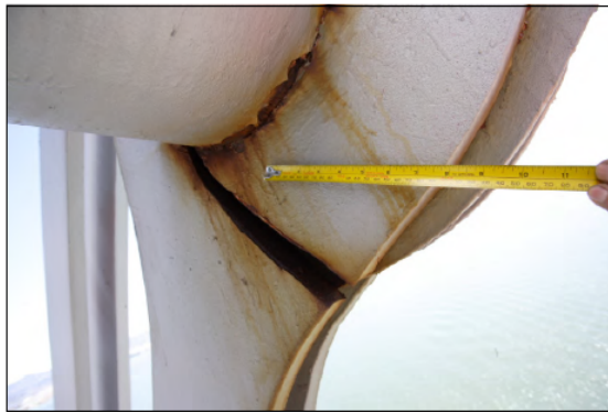
Figure 5. Example of eyebar showing crack and failure location. Reproduced from [21].
