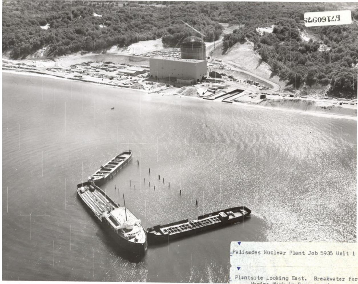
Figure I-11 A Photograph from June 1968, Looking South over Palisades Nuclear Plant Site. Note the Cleared Vegetation and Road Cut into the Sand Dune to the Right of the Reactor Vessel Building and the Land Grading and Vegetation Clearing along the Beach to the South of the Site. Source: HDI 2024-TN10670.
