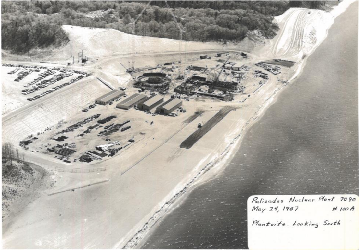
Figure I-10 A Photograph from April 25, 1967, Looking Northeast over Palisades Nuclear Plant Site. Note the Cleared Vegetation and Road Cut into the Sand Dune to the Right of the Circular Footprint of the Future Reactor Vessel Building and the Land Grading and Vegetation Clearing along the Beach to the South of the Site. The Original Photograph Caption States, "The lake is washing sand from the south disposal area." Source: HDI 2024-TN10670.
