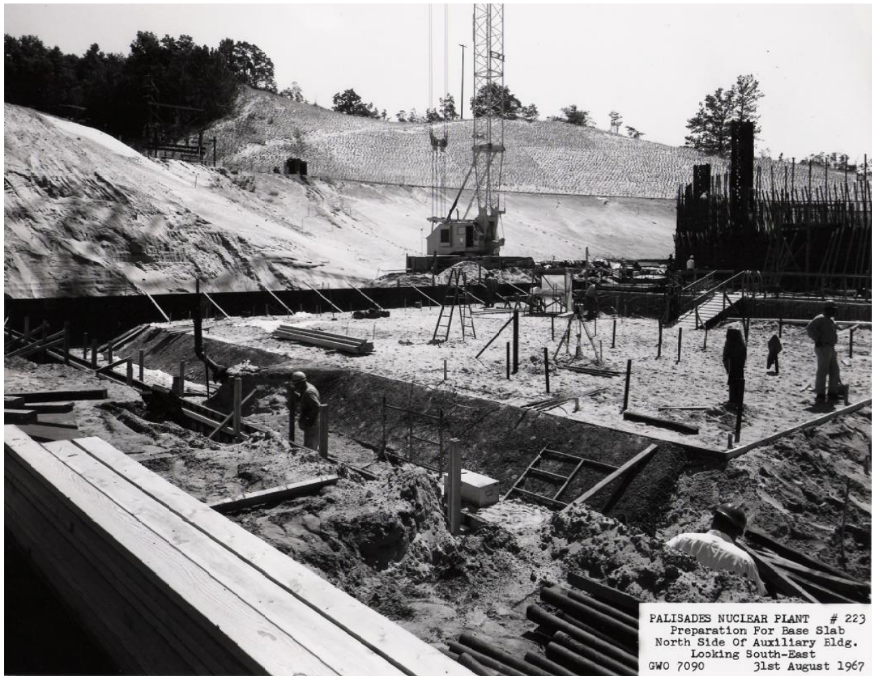
Figure I-12 A Photograph from August 31, 1967 Looking Southeast from the Auxiliary Building Foundation of Palisades Nuclear Plant. Note the Cleared Vegetation and Road Cut into the Sand Dune behind the Crane. The Existing Transmission Pole on Top of the Sand Dune Is Located Where the Current Transmission Lines and Structures Are Located Today. The Sand Dune Has Already Undergone Revegetation. Source: HDI 2024-TN10670.
