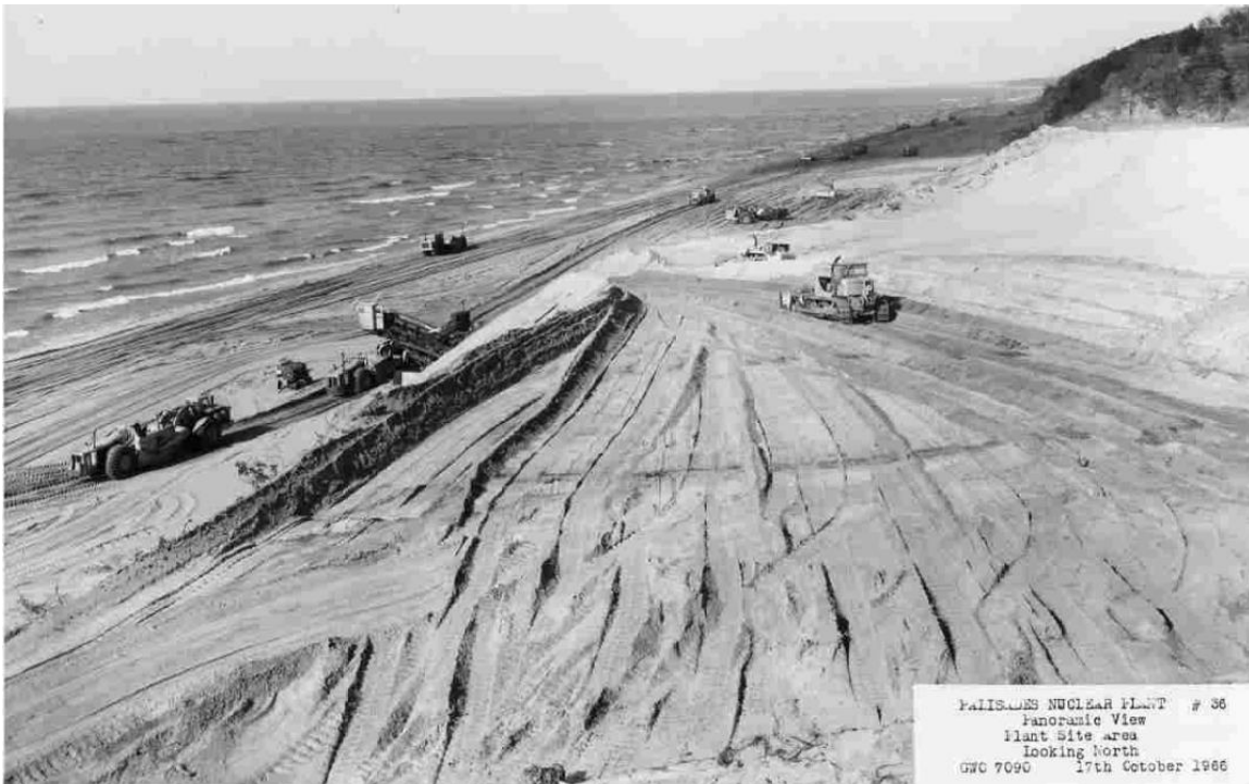
Figure I-5 Heavy Equipment Grading the Beach at the Palisades Nuclear Plant Site on October 17, 1966. Photograph Looking to the North. Source: HDI 2024-TN10670.
