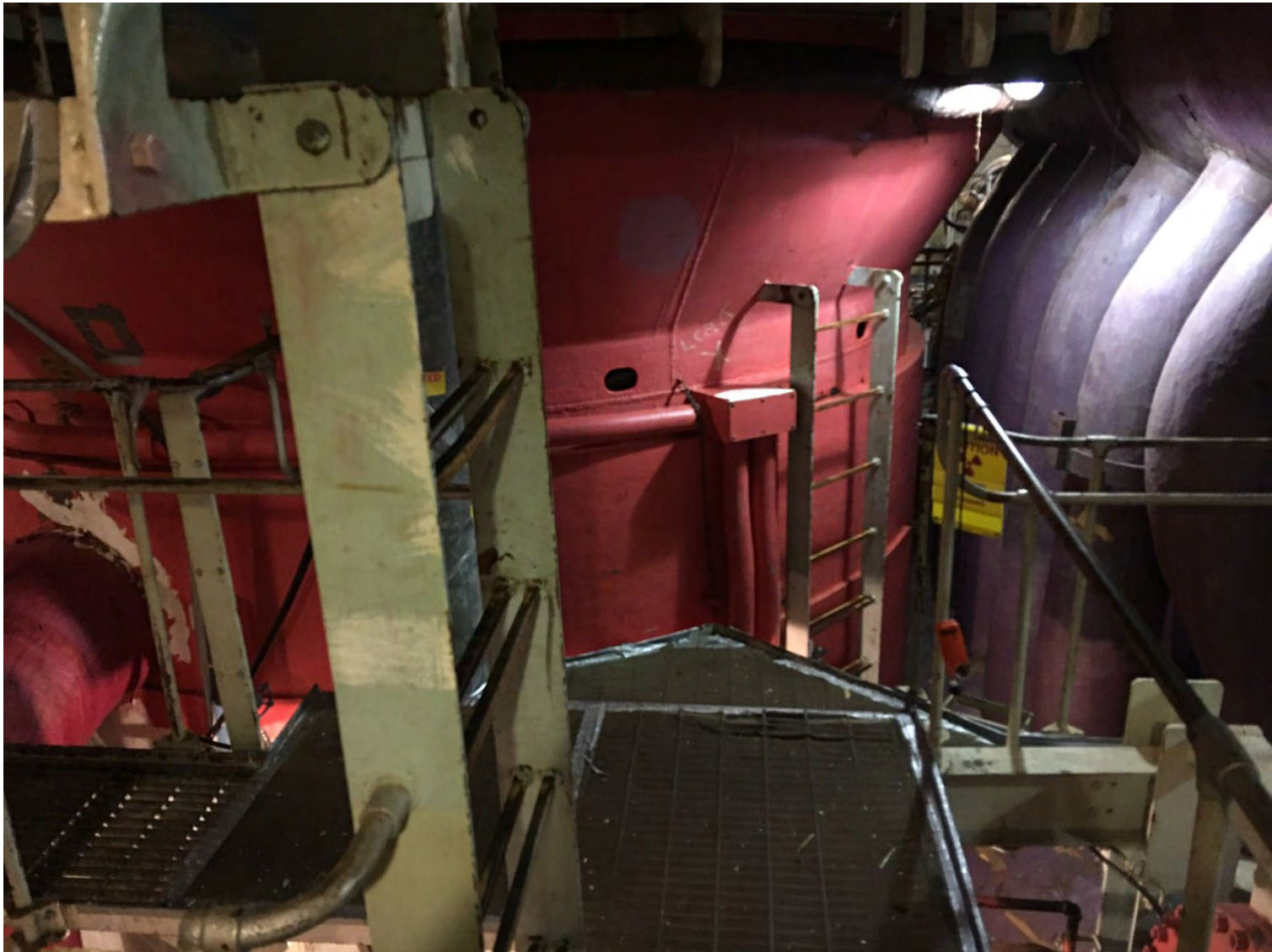
Containment Vessel – Before
