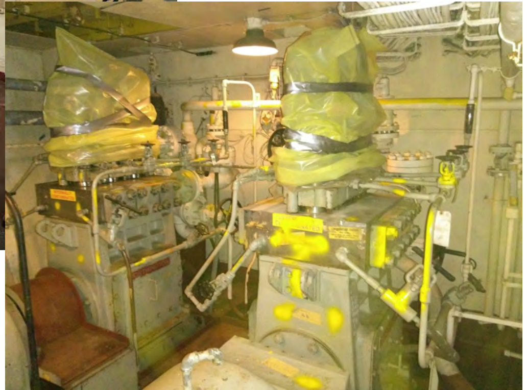
Charge Pump Rooms – Before and After
