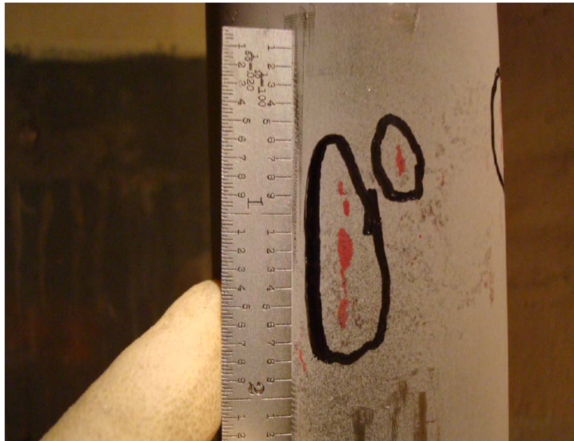
Figure 3-6 Example of CISCC under a pipe hanger in an ECCS piping section. The pipe hanger provides a concentrating mechanism for chloride entrapment, producing cracking in locations that are not accessible for visual inspection. (PNNL presentation on CISCC)
