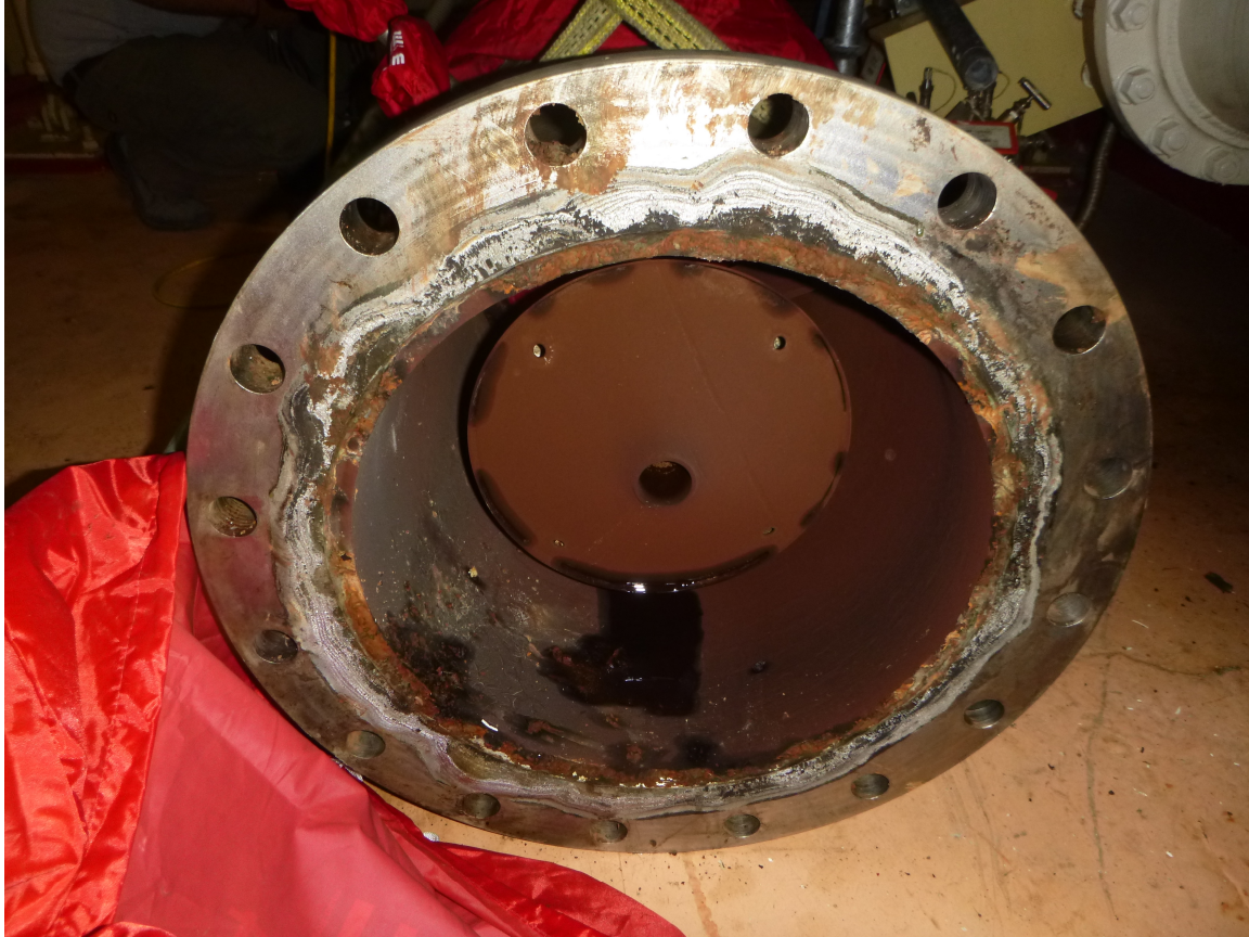
Figure 3-5 Flow element flange with severe crevice corrosion (courtesy Exelon).
