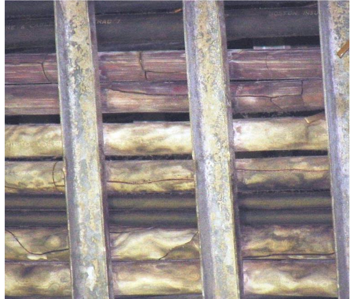
Thermal degradation showing that cables age based on both the environment and by polymer type. The cracked cable jacket is chloroprene; the black cable jacket is chloro-sulfonated polyethylene.
