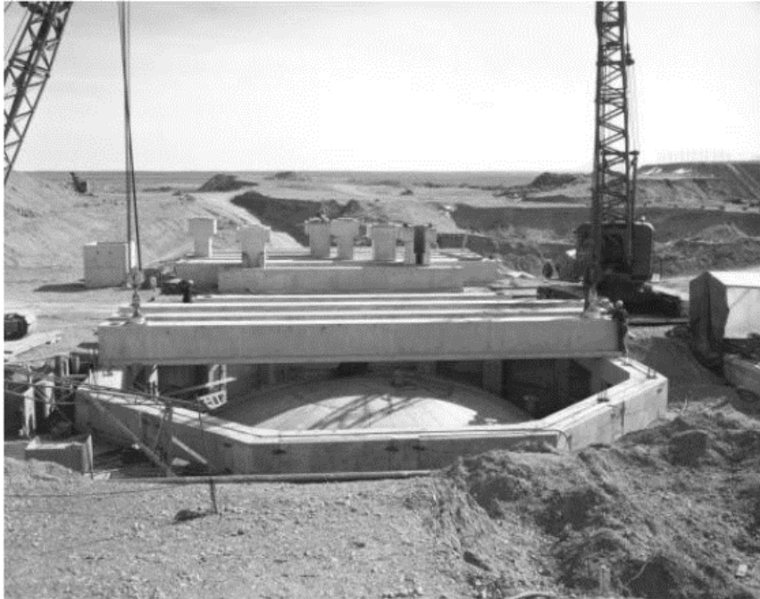
Figure 3-2. Pillar and panel octagonal vault for tank WM-185 showing concrete beams and concrete risers (DOE, 2003)
