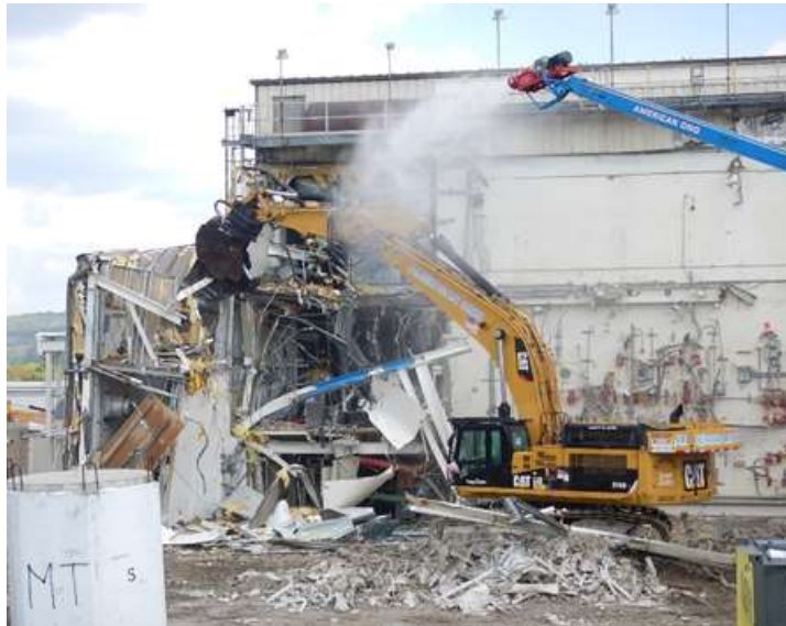
Dust Suppression Equipment Previously Used At WVDP
