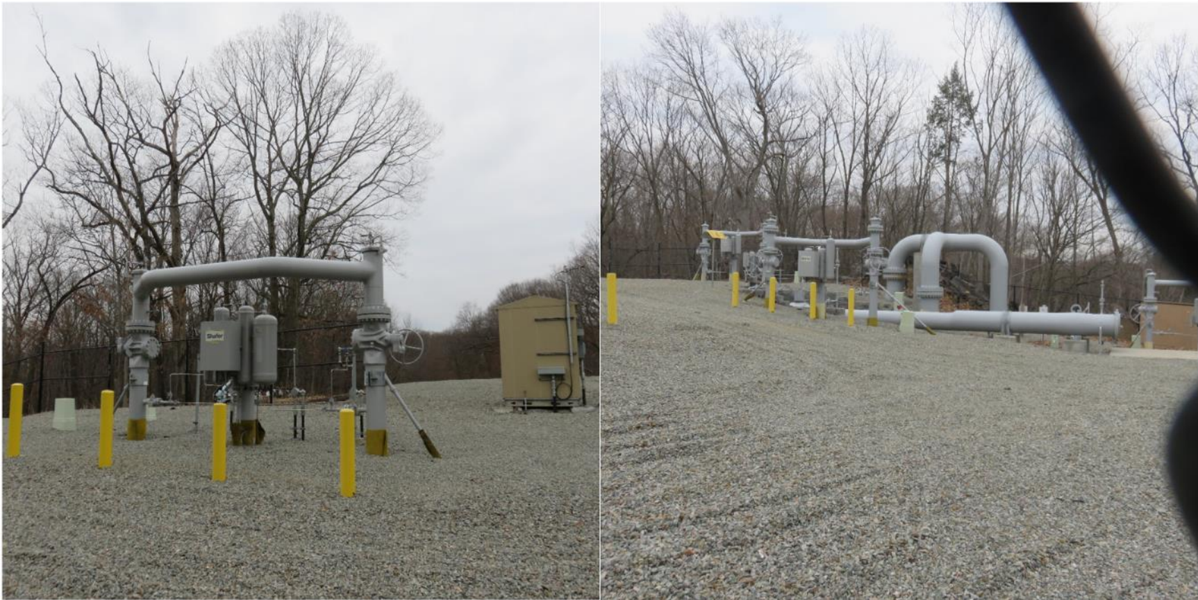
Figure 6. Images of above-ground connections where the 26-inch, 30-inch, and 42-inch pipelines connect, east of Indian Point. These photos were taken by the team on March 12, 2020.
