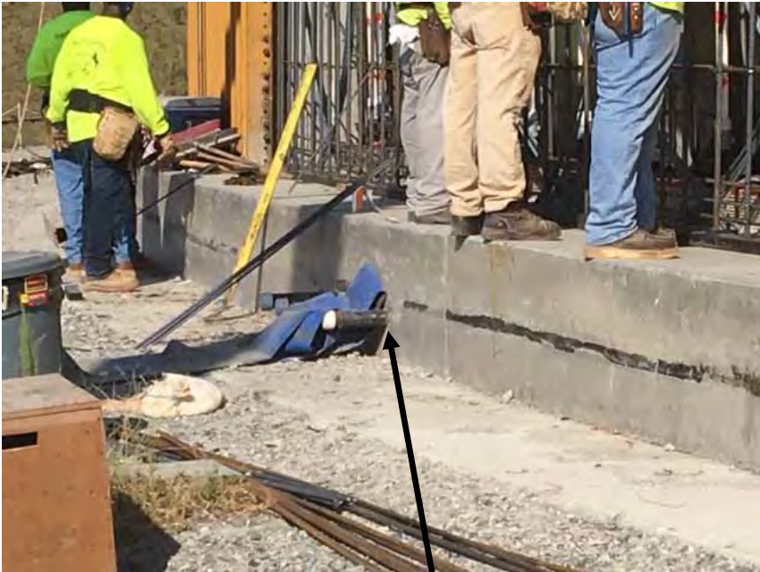
Shotcrete Piping - Exterior
