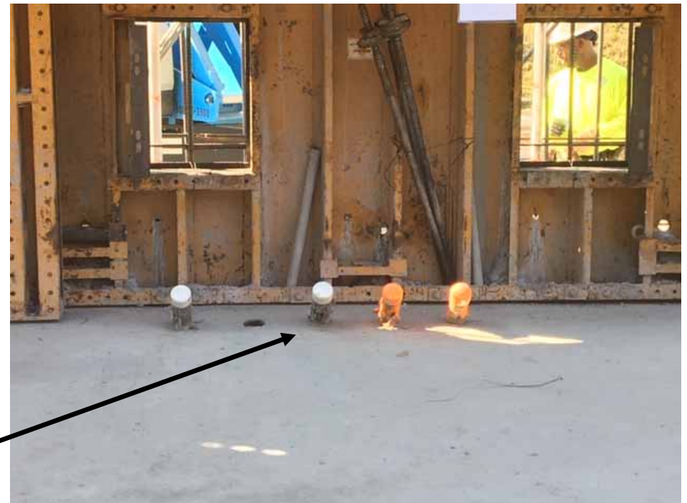
Shotcrete Piping - Interior
