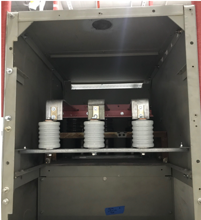
KEMA HEAF test switchgear Al bus bars, 11.5 cm gap
