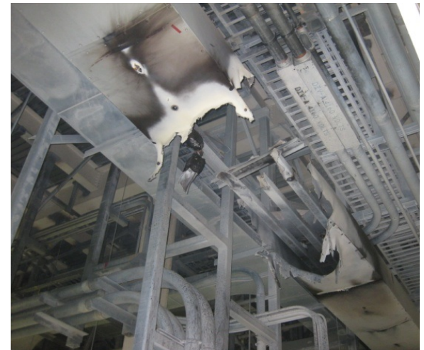
Columbia Bus Duct (OpE) 2009
