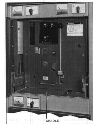
Fig. 4 Type DS-206 Breaker in Connected Position (392506)
