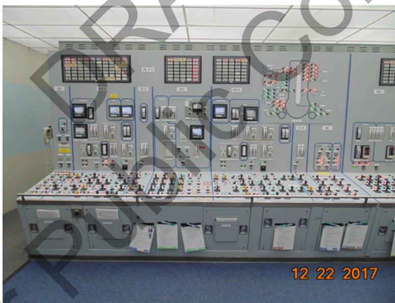
Figure 8-7 Example 2: Main Control Board Sections 9-3 and 9-4
