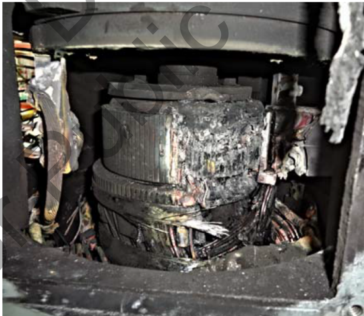
7 8 Figure 5-12 9 40 hp Motor Fire Event – Internal Impacts
