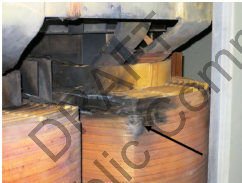
Figure 5-22 Damaged Dry-Type Transformer [43]
