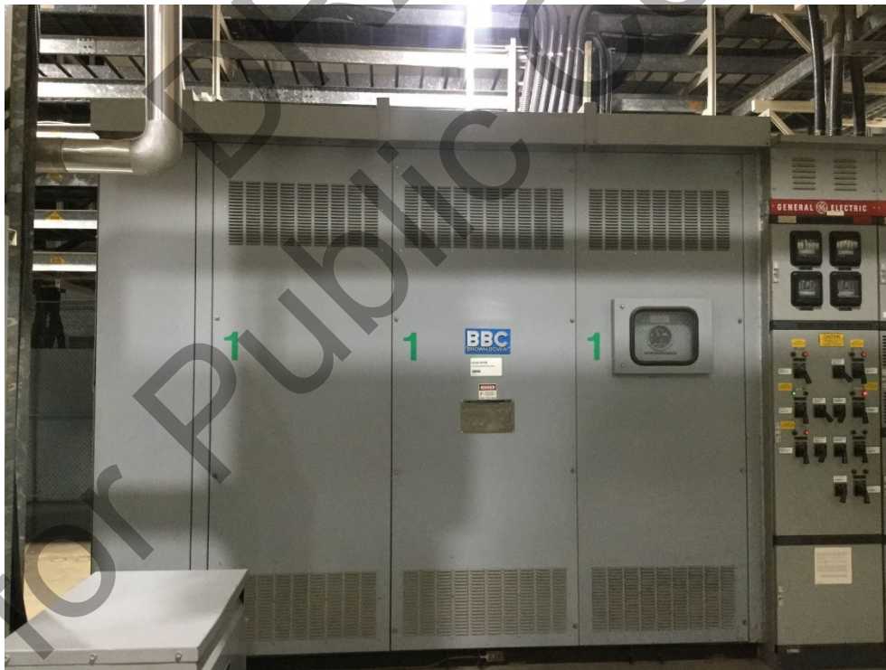
Figure 5-16 Example of Typical Large Dry-Type Transformers (2000 kVA)
