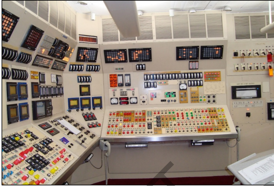
Figure 8-3 Example 1: Main Control Board
