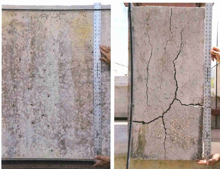
Confined Face of ASR-affected Beam (left); Unconfined face of Same ASR-affected Beam (right)
