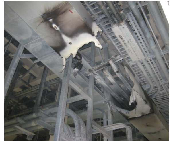
Columbia Bus Duct (OpE) 2009
