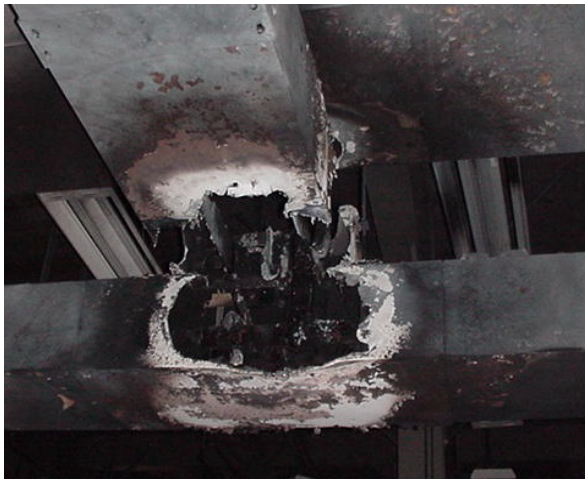
Diablo Canyon Bus Duct (OpE) 2000
