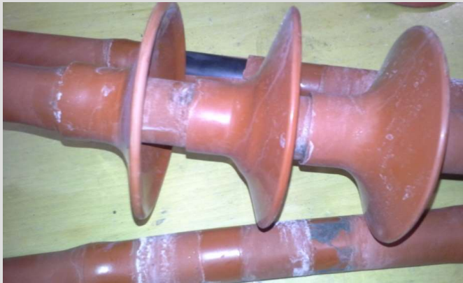
Tracking and erosion insulator shed
