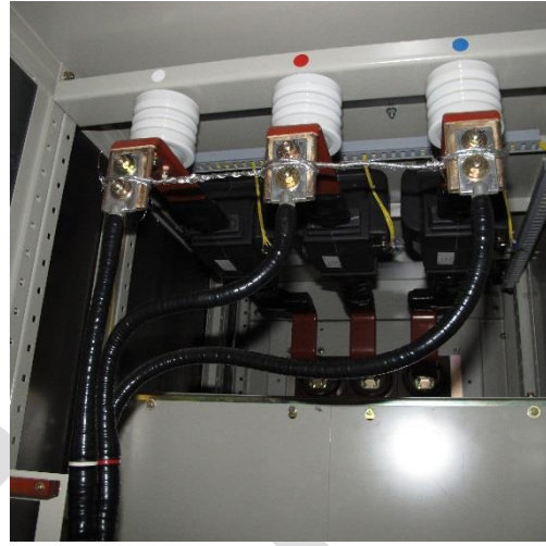
Figure 6. Example arcing wire location.
