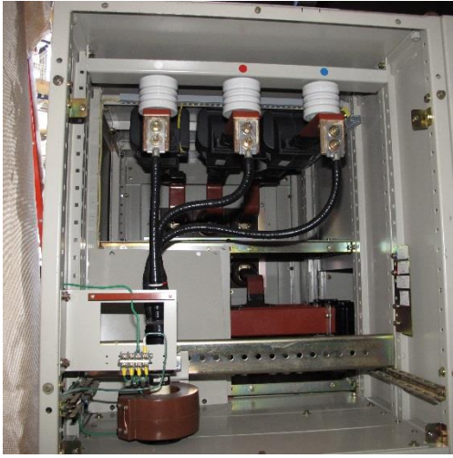
Figure 5. Electrical cabinet bus bar example.
