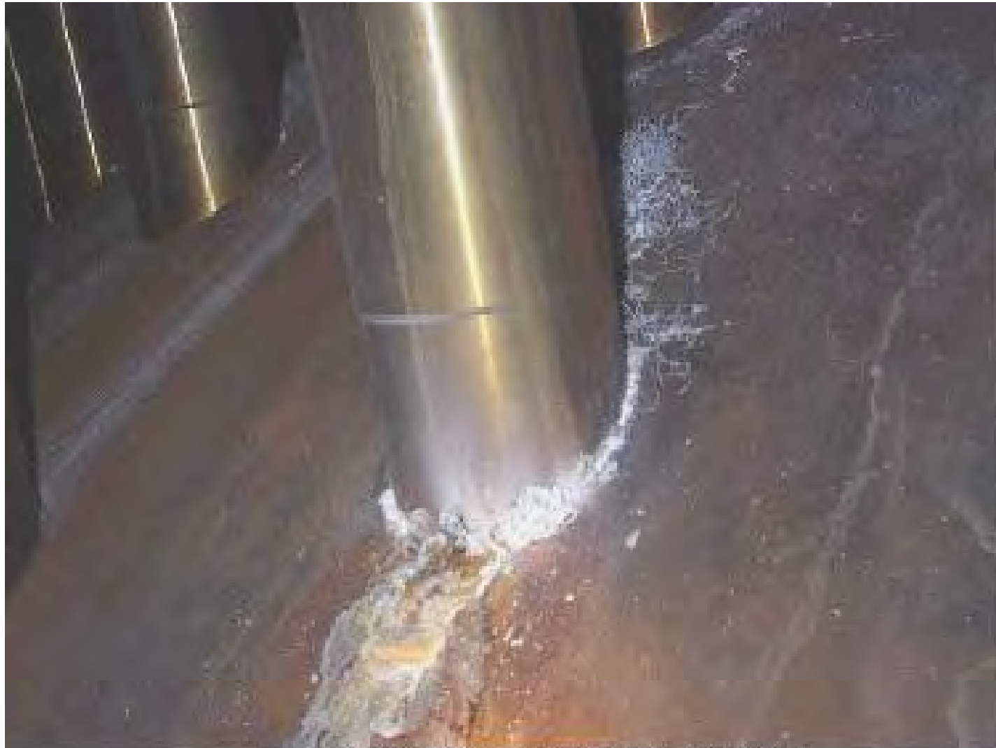
CRDM Nozzle Leakage Observed at Oconee 3
