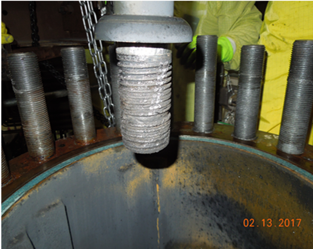
Figure 1: As Found Pictures of Failed Unit 2 HPCS Injection Valve Stem to Wedge Connection
