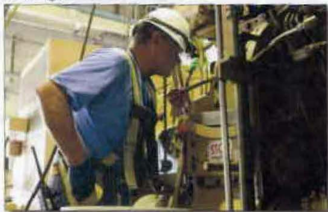
Maintenance removed the governor from the "A" emergency diesel generator yesterday and has disassembled the component in the shop.
