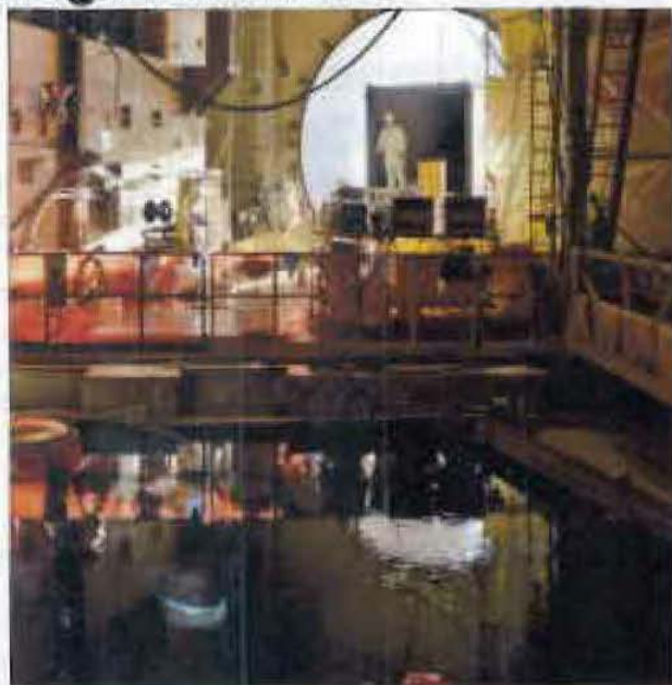
Crews are working to demobilize equipment and scaffolding as work projects wrap up inside containment.
