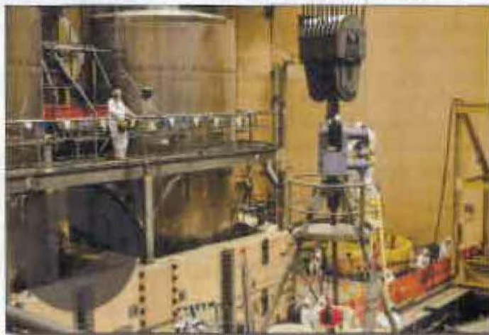
Members of the head area maintenance team prepare for the reactor vessel head lift late yesterday morning. Click on the picture above to view a time-lapse video of the lift.
