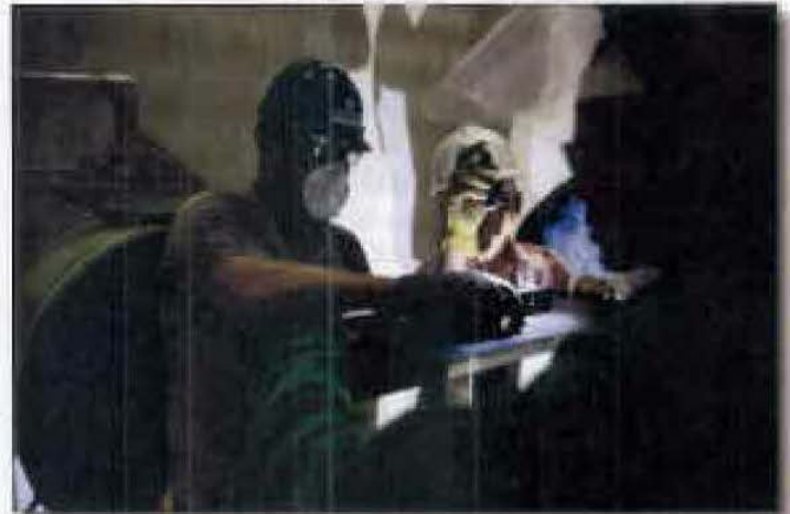
Day & Zimmermann crews work to install a support structure in the essential service water pumphouse for a FLEX modification.
