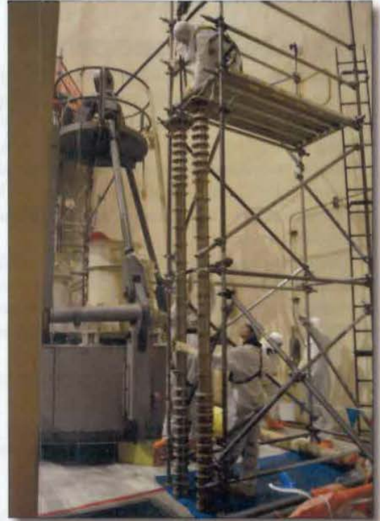
The Emergent Issues Team is working a plan to remove control rod drive mechanism coil stacks and dummy cans on spare penetrations to address the reactor head issues.
