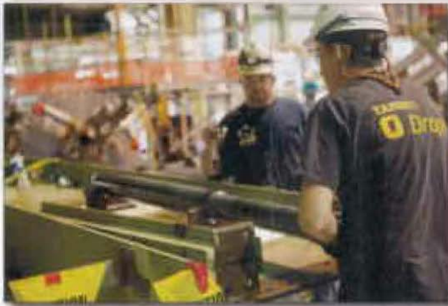
While the critical path work is all inside containment, there is a lot of important work going on elsewhere, including on the turbine deck.
