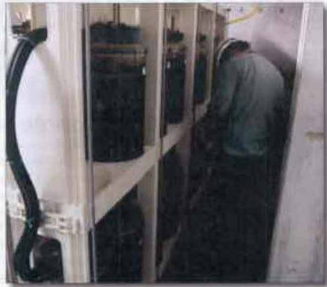
Electrical Maintenance performed impedance testing on the NK014 battery cells to verify the individual cells are within the tech spec requirements to satisfy operability
