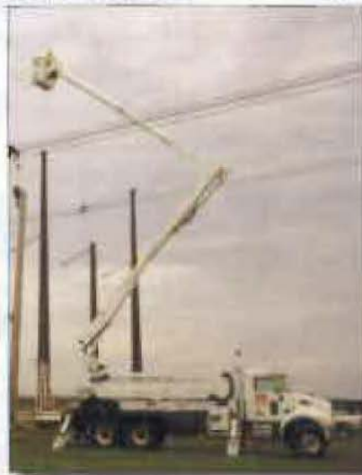
The switchyard reliability upgrade team is in the process of moving the Waverly/LaCygne line.
