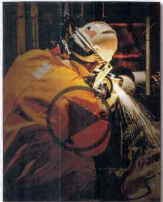
Work is progressing well on the essential service water (ESW) piping replacement to the containment coolers. Click the image above to view a time lapse video of insulation being installed.
