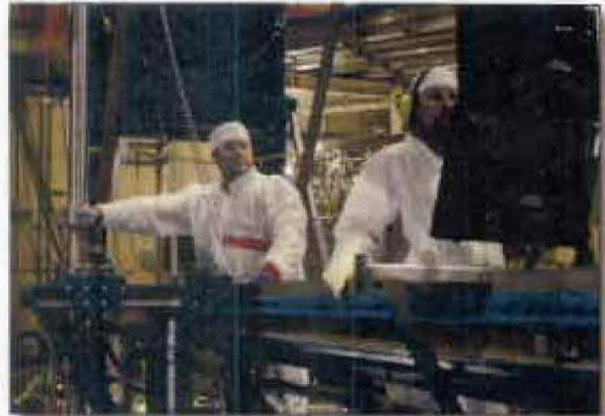
The non-destructive examination of the reactor vessel bottom nozzles continues.
