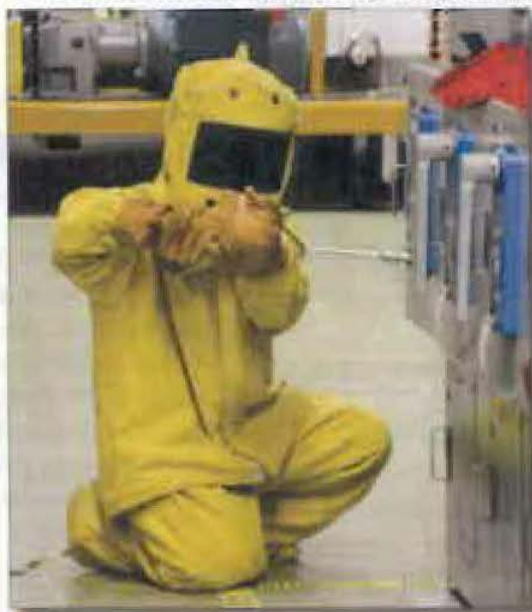
Maintenance completed PG19 load center work ahead of schedule, allowing the polar crane to be returned to service earlier than expected. Jessica Doidge, nuclear station operation, energizes the breakers.
