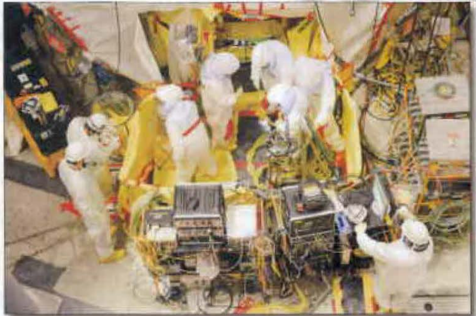
The team today completed ultrasonic volumetric testing of the 12 selected nozzles under the reactor head. Canopy seal clamps #77 and #11 have been installed and #23 is being installed today.
