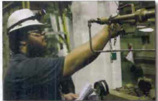
Wis Houston, Jr. walks down the clearance under in preparation to start work on the "A" emergency diesel generator.
