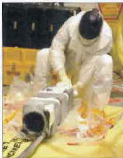
Removal of boric acid from the reactor vessel head, CRDM and DRPI coil stacks continues in containment.
