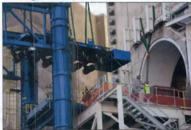
Yesterday, personnel lifted the self-propelled modular transporter to the deck of the equipment hatch.
