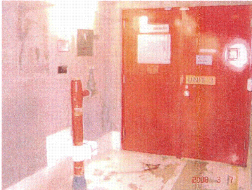
Fire Riser just outside SFP (Elev 63'-6")
