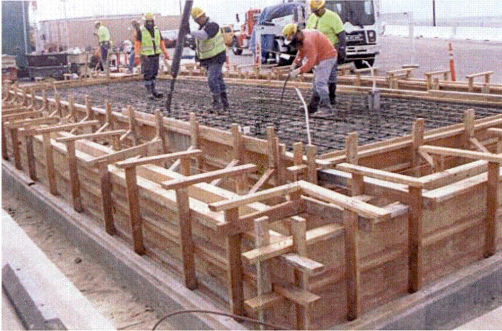
1500 KW Standby Generator - Base
