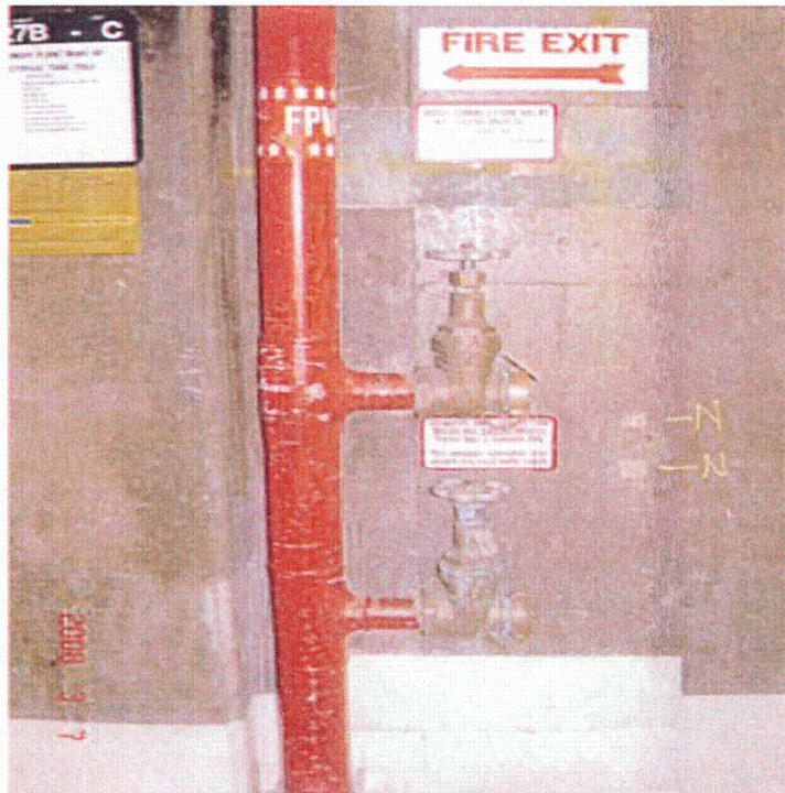
Fire Riser just inside of the door (to the outside at Elev 37')
