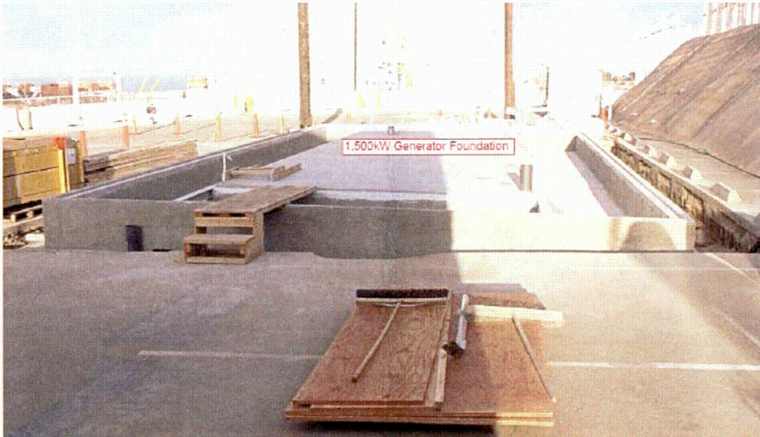
1500 KW Standby Generator - Base
