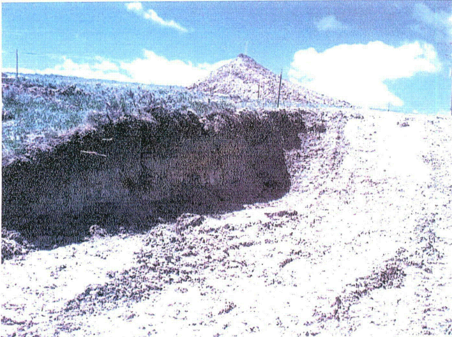
Figure 2 Steep cuts with no sediment control in Mine Unit K North
