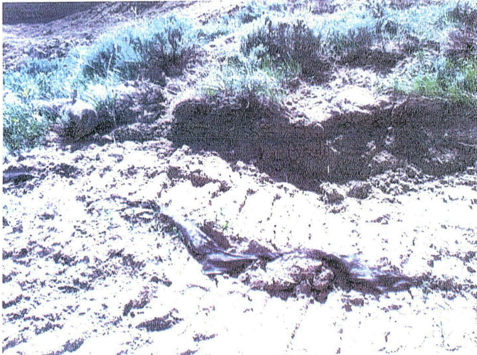
Figure 4 Abandoned silt fence and erosion in Mine Unit K North
