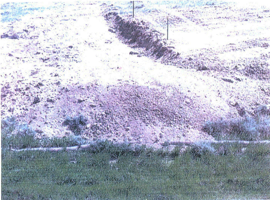
Figure 3 Sediment over-topping straw wattles in Mine Unit K North
