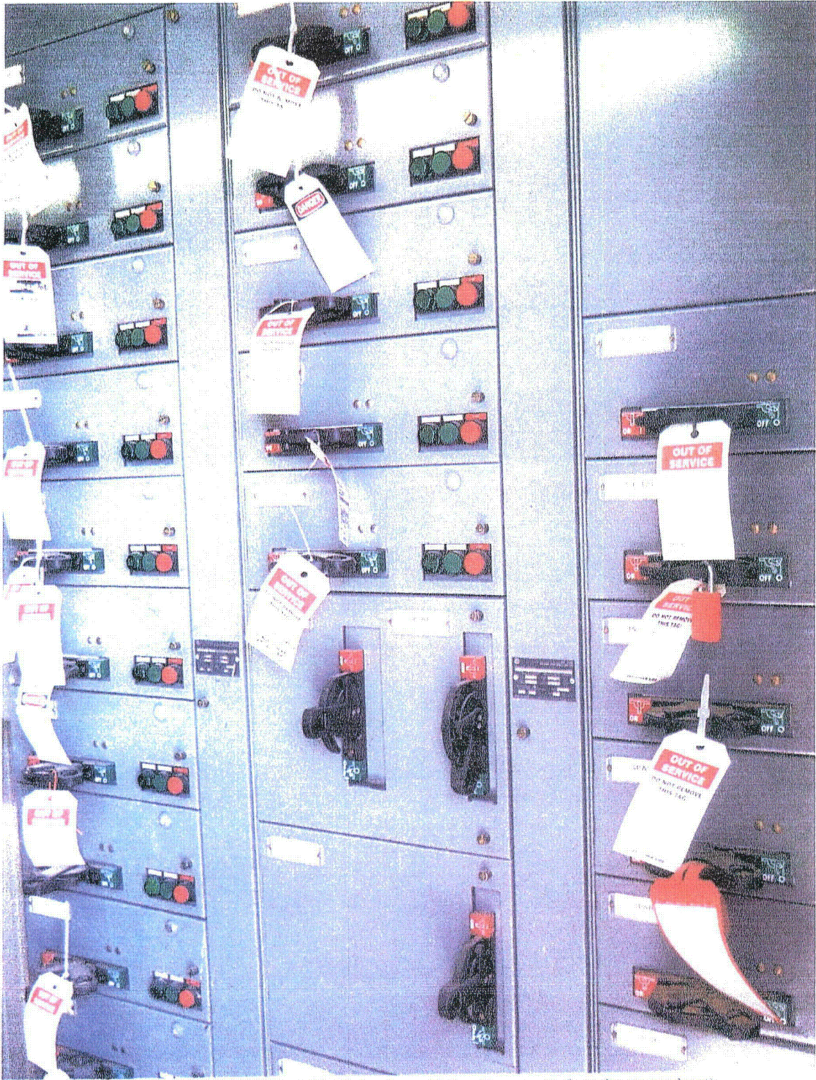
Figure 15 Panel inside a header house in MU-15 showing which wells are out of service (tagged out)
