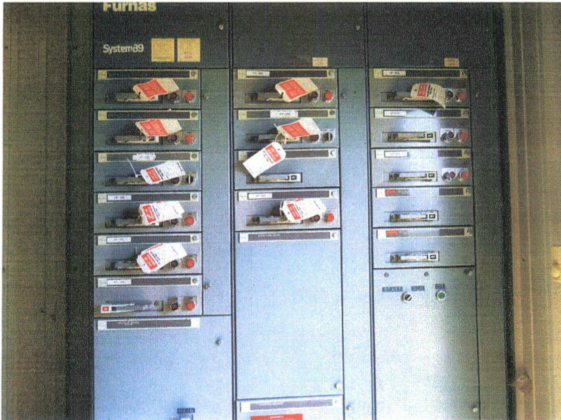
Figure 20 Panel in MU-H header house showing many wells tagged out.
