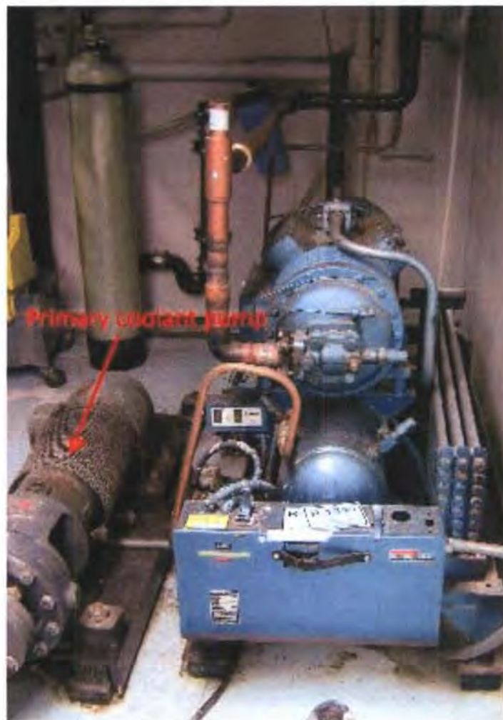
Figure 5.2-3 Primary coolant pump system
