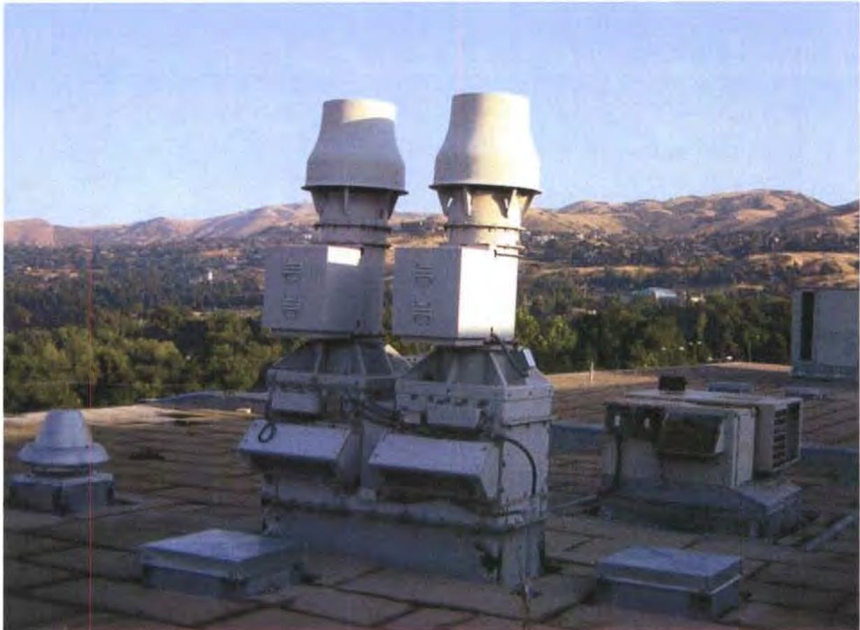
Figure 9.1-2 Two exhaust motors for the UNEF ventilation system
