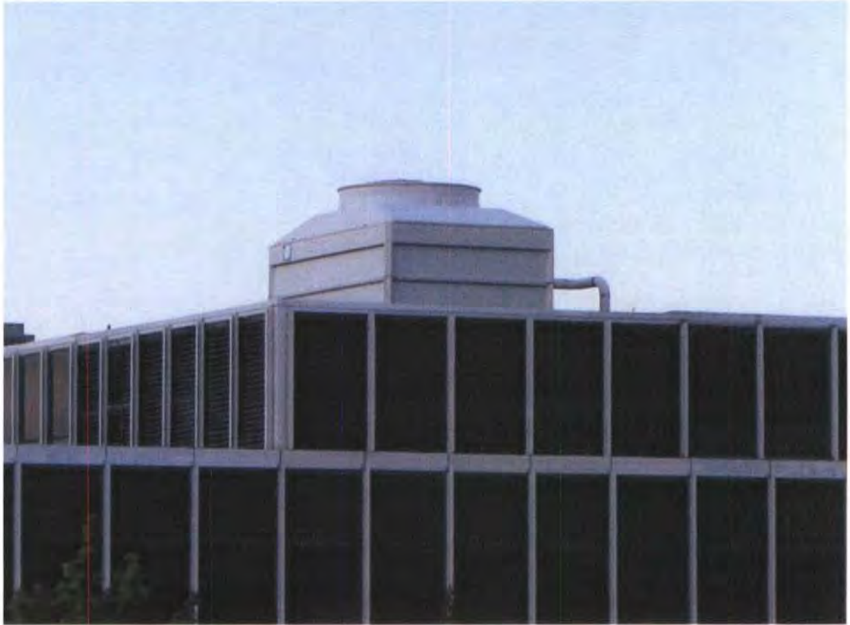
Figure 9.1-1 The cooling tower for the MEB HVAC system
