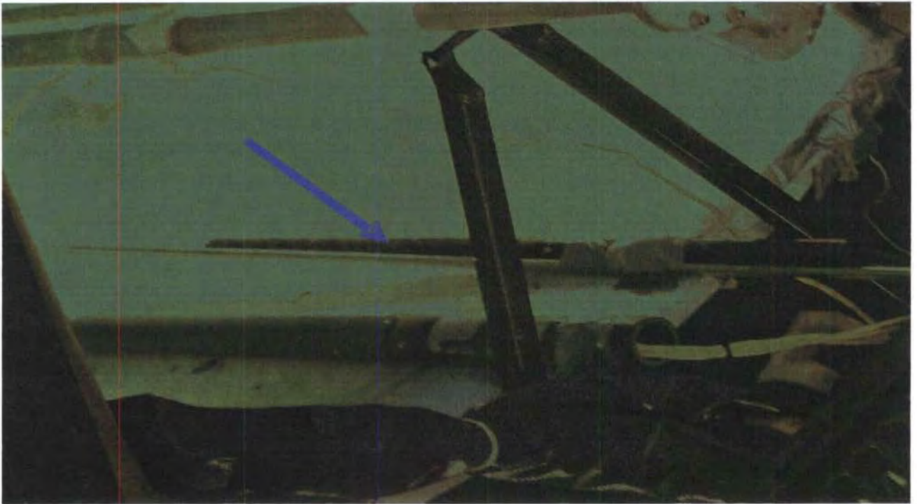
Figure 5.4-3 In-tank pH meter (indicated by arrow)
