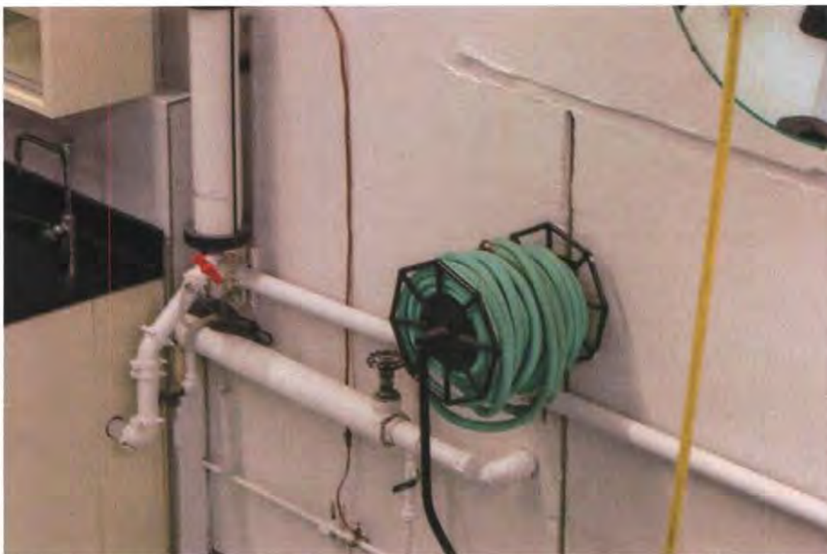
Figure 5.2-2 Emergency water supplier in the reactor room
