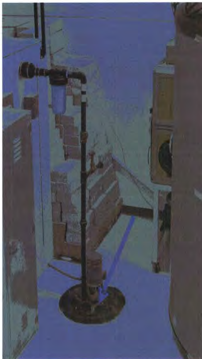
Figure 5.4-5 A 40-gallon water storage (indicated by arrow)
