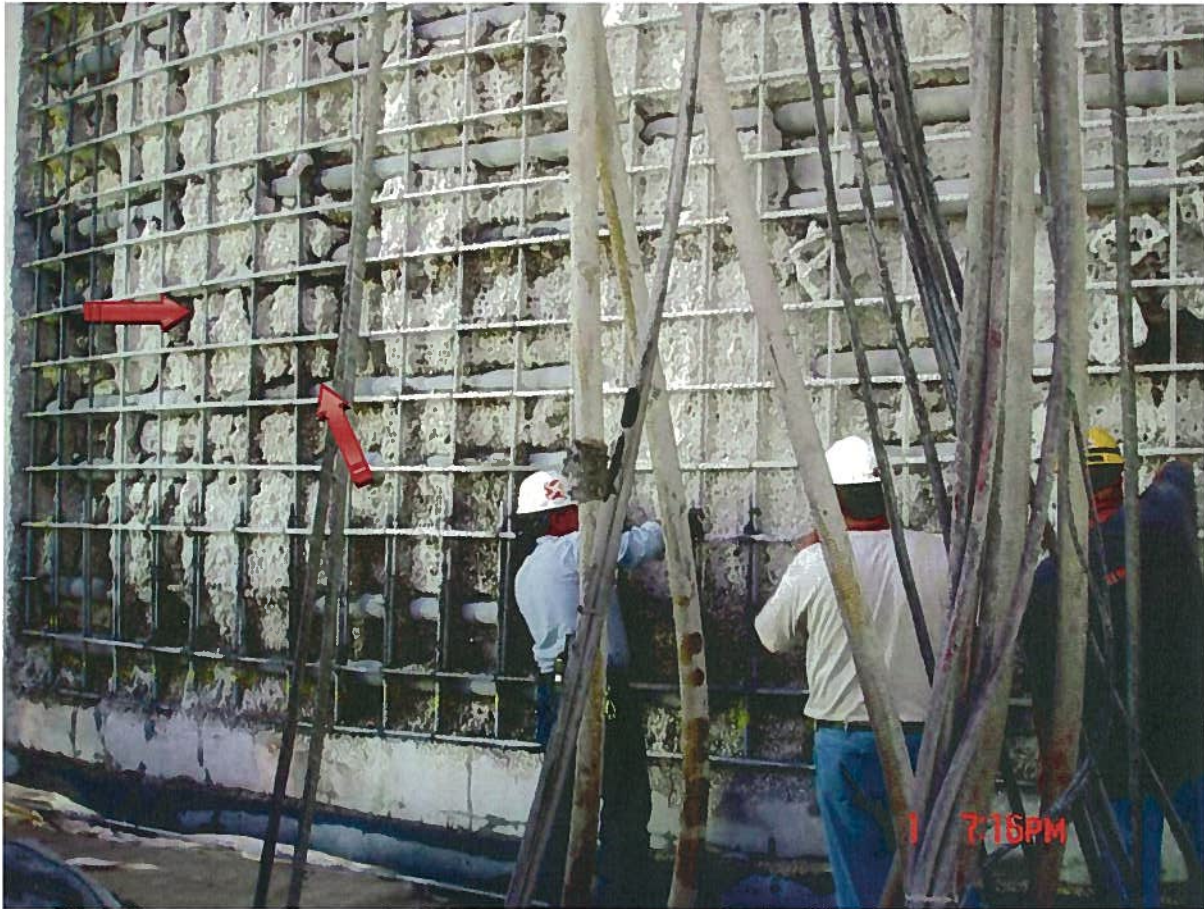
Figure A4.4 Photograph of demolition on the evening of 10/1/09. Note the large blocks of broken concrete in the middle of the opening.
