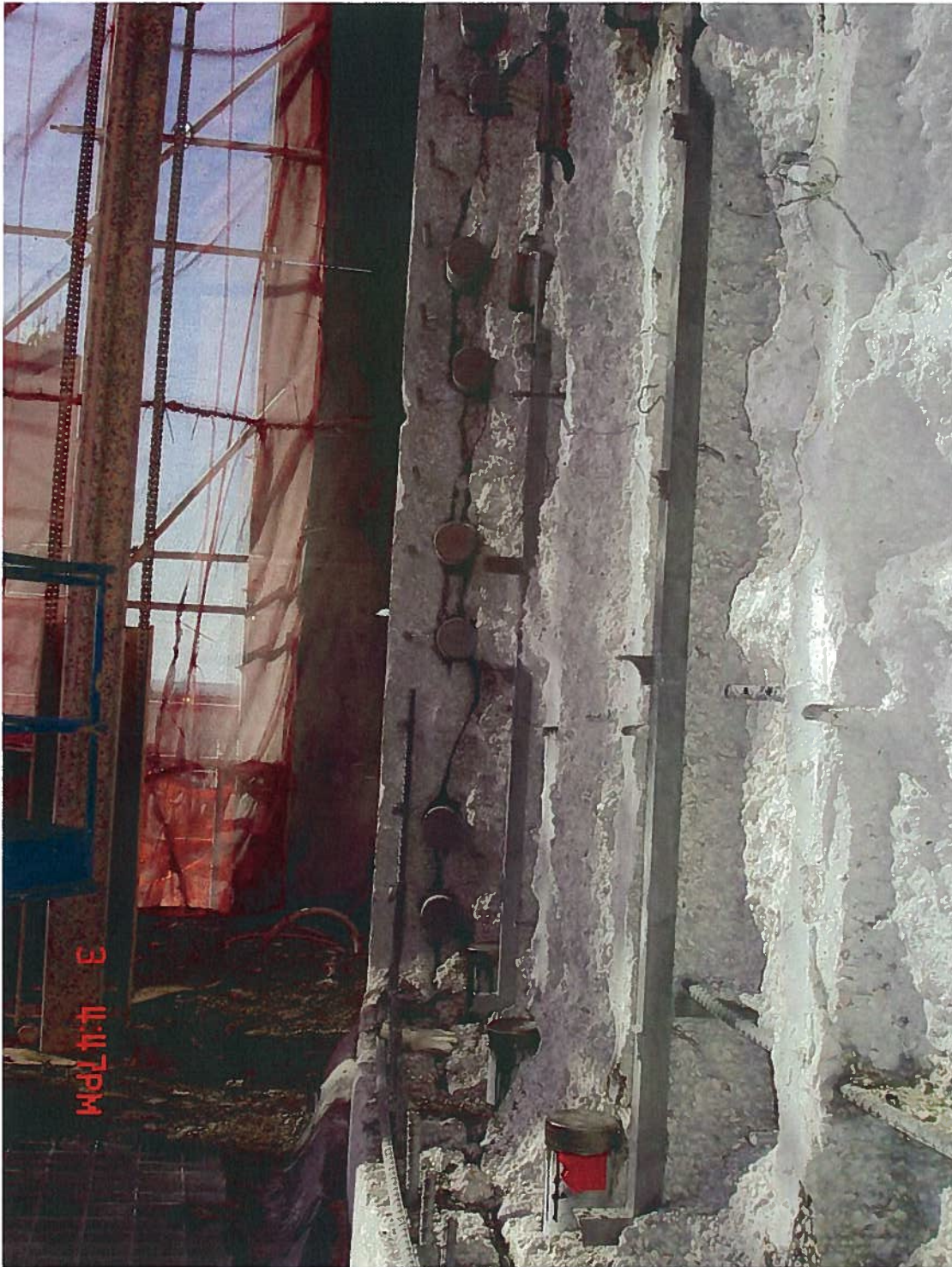
Figure 1.3 Photograph of delamination crack running from horizontal tendon to horizontal tendon, parallel to the wall surface, approximately 10 inches deep. (Photo taken after partial concrete demolition)
