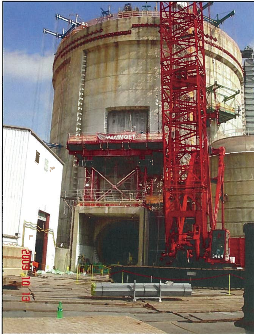
Figure 1.1 Photograph of the steam generator opening worksite. Note the newly constructed rectangular opening above the existing circular equipment hatch.
