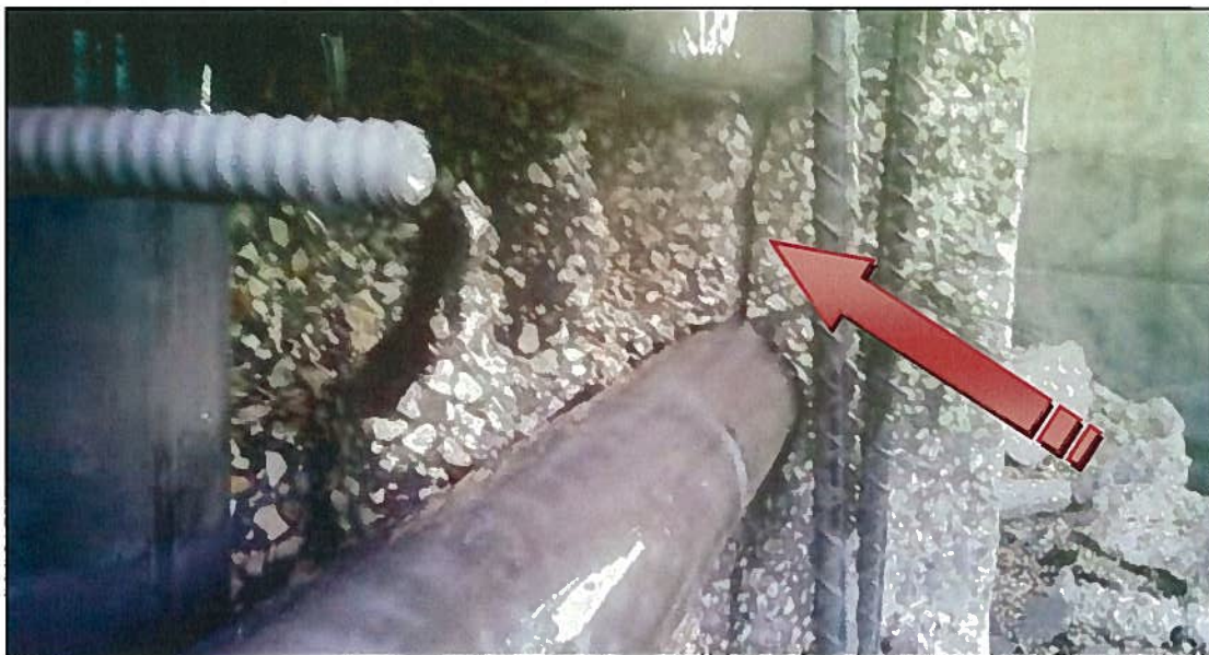
Figure A4.3 Another crack photograph taken on 10/01/09
