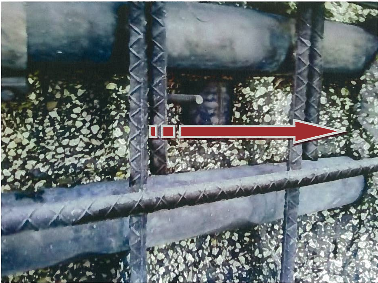
Figure A4.1 The first indication of cracking between horizontal tendons taken on 9/30.
