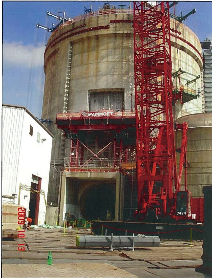
Figure 1.1 Photograph of the steam generator opening worksite. Note the newly constructed rectangular opening above the existing circular equipment hatch.
