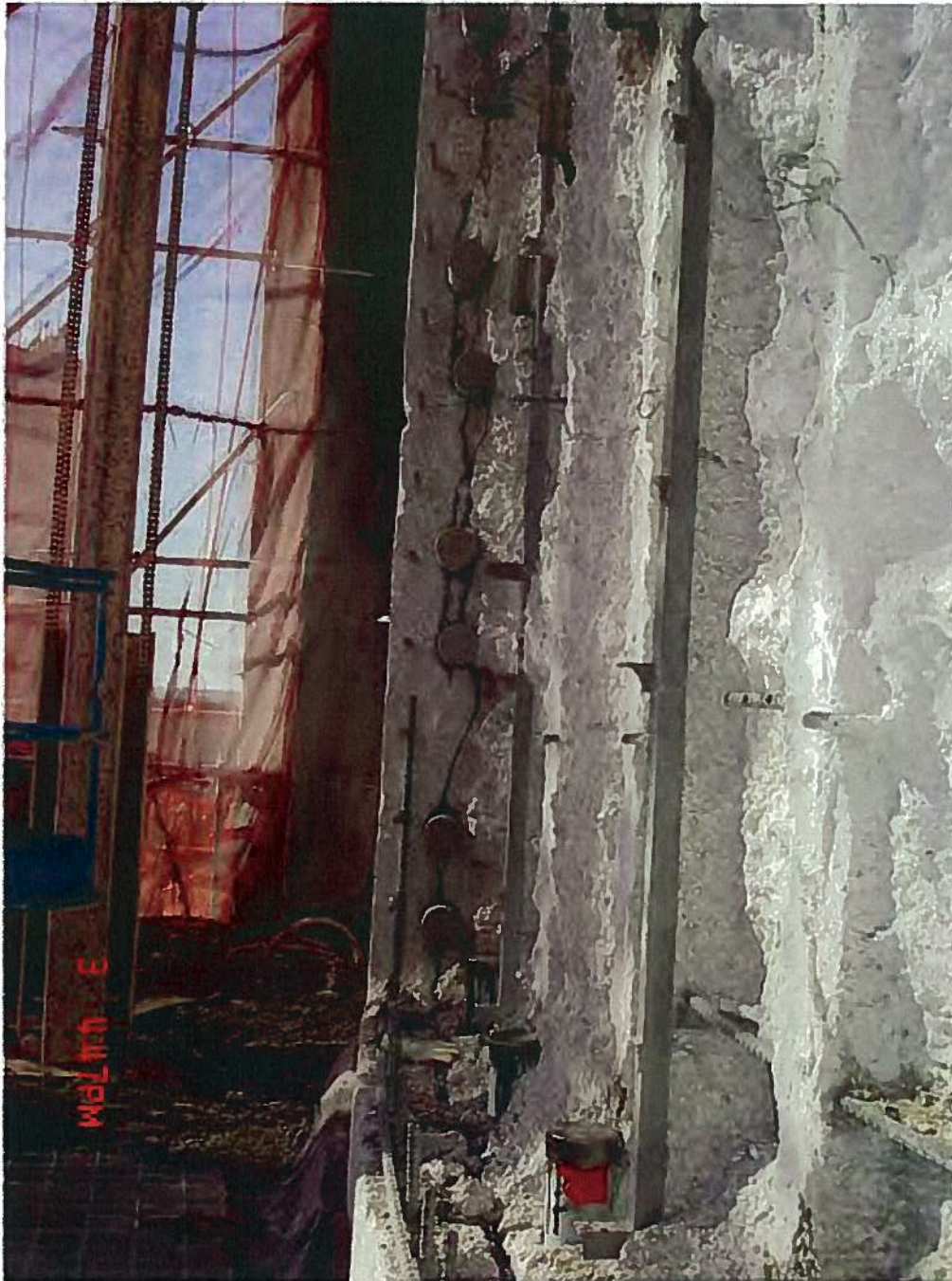
Figure A4.6 Delamination crack running vertically between horizontal tendons about 10" deep. Taken on 10/3/2009
