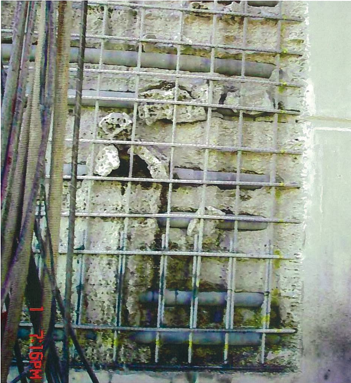
Figure A4.5 Another early photograph (10/1/09) of concrete debris, showing the distribution of horizontal tendons. The horizontal tendons come in pairs centered 13 inches apart. The distance between pairs is 26 inches. The horizontal tendons are outside the vertical tendons and define the transition from radial tension stress to radial compression stress in the concrete.
