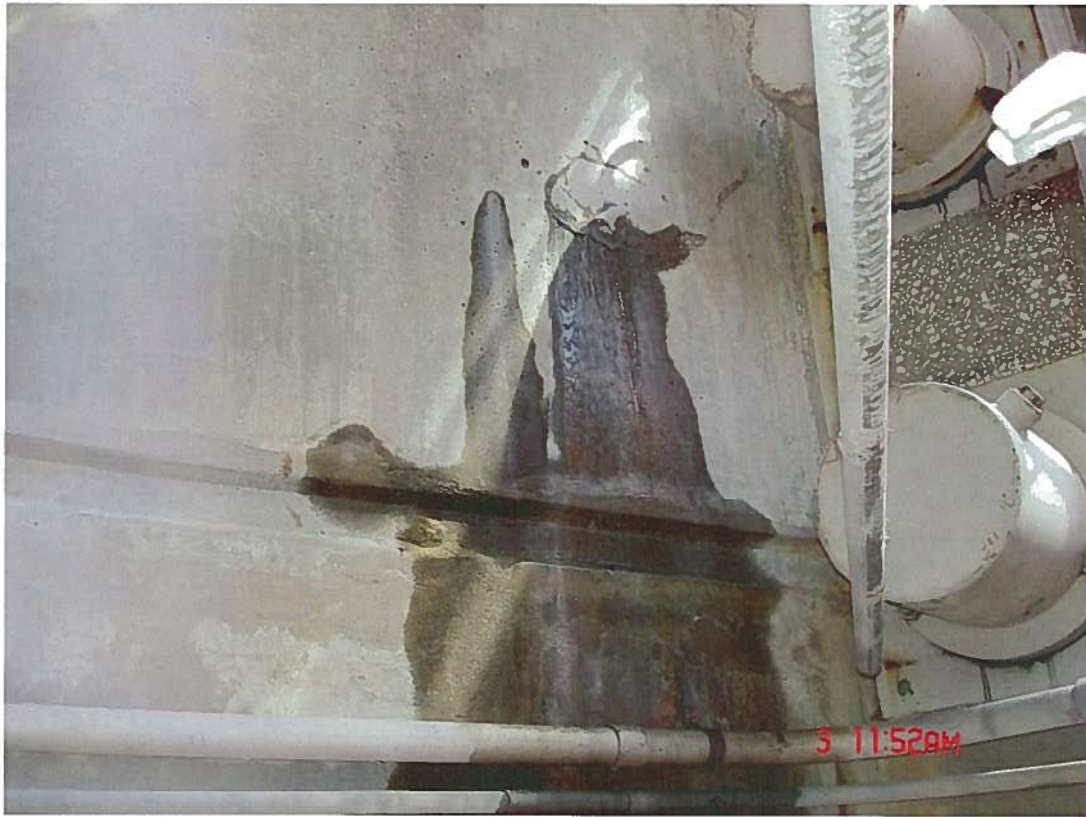
Figure 1.2 Photograph of water leakage from the containment wall (10/3/2009).
