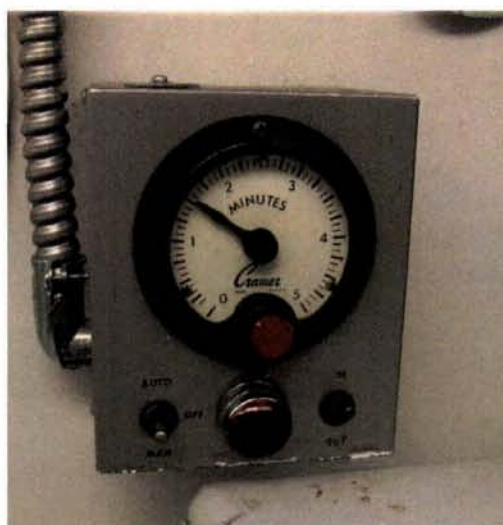
Figure 10.7 Pneumatic Transfer System Controller
