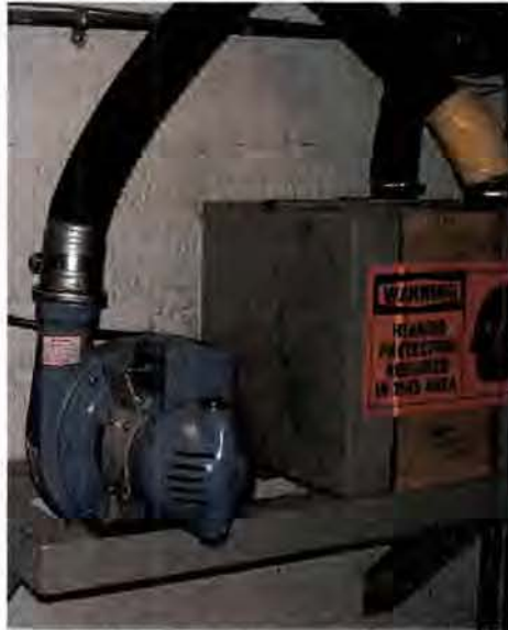
Figure 10.8 Pneumatic Transfer System Blower-and-Filter Assembly
