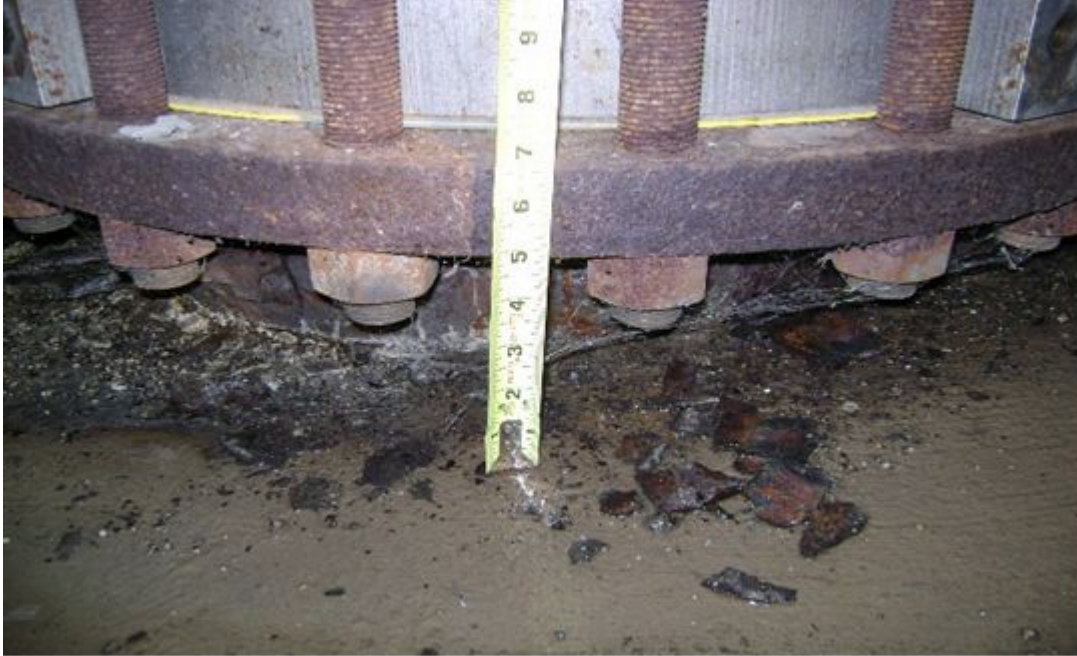
Picture No. 1 - 0A SX Riser Pipe – October 19, 2007
