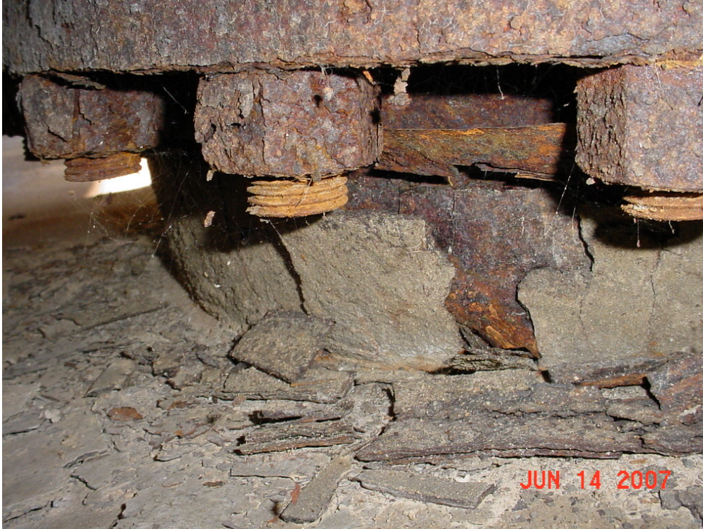
Picture No. 5 – 0E SX Riser Pipe- June 14, 2007
