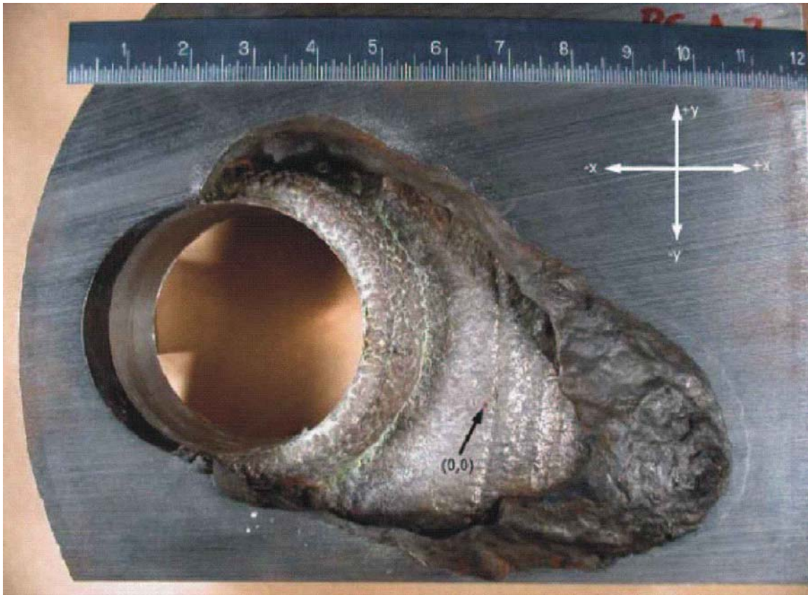
Fig. 1. (continued) (c) sketch of RPV head degradation; and (d) photograph presenting a plan view of the wastage-area footprint showing remaining J-groove weld, irregular topography of exposed unbacked cladding, and irregular sidewalls of the wastage cavity [7].
